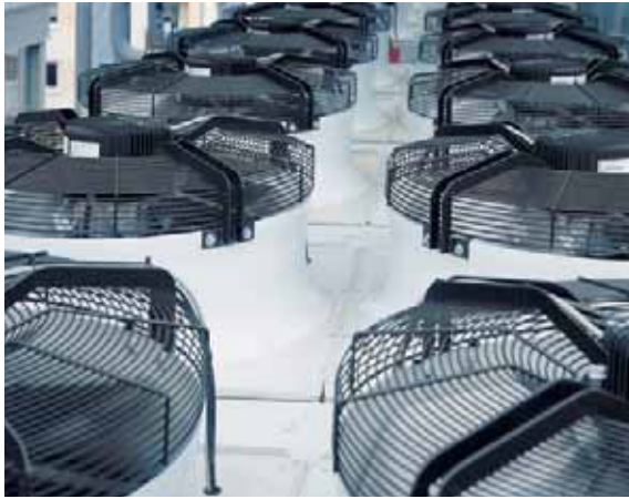
80 large EC fans on the roof deliver the required heat exchange.
